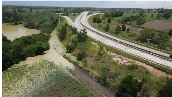
Fig. 1. Landslide on the Terpeka Toll Road Access to Gunung Batin Sta. 1+300
