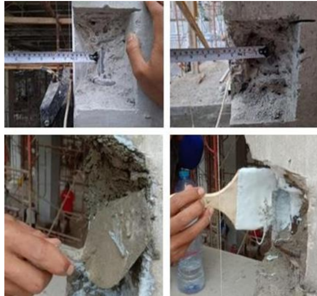
Fig. 4. Segregation and Porous Beams
