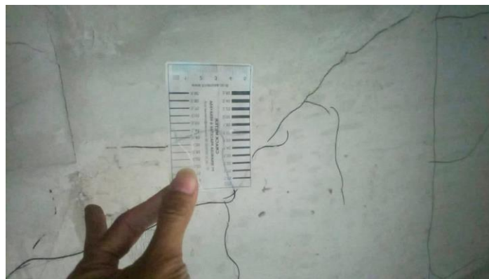
Fig. 6. Examples of Cracks in Beams in the Structure of RSUD X Bandung
